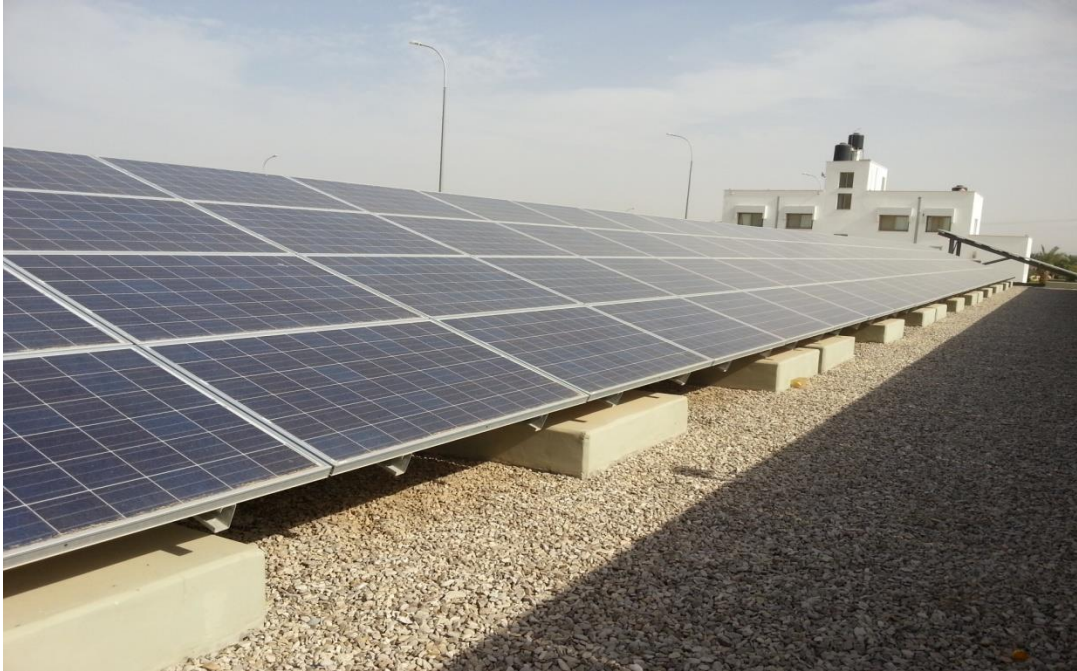
Figure (3.6): Solar panels in Jericho WWTP
