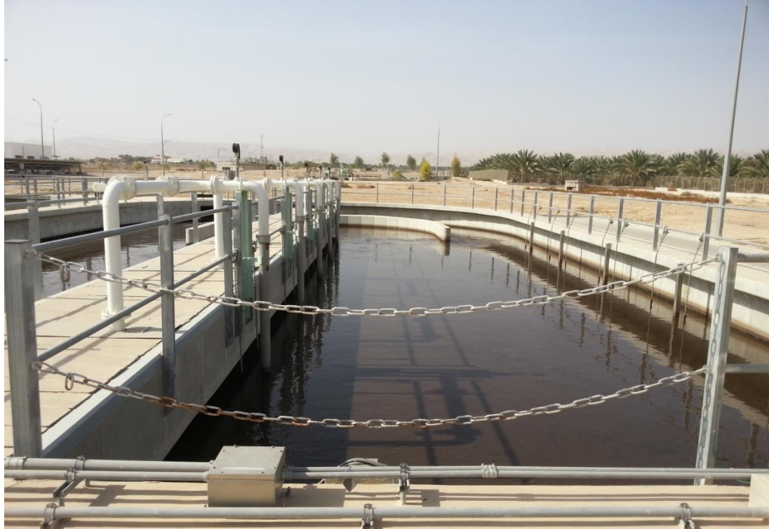
Figure (3.4): Reactors in Jericho WWTP
