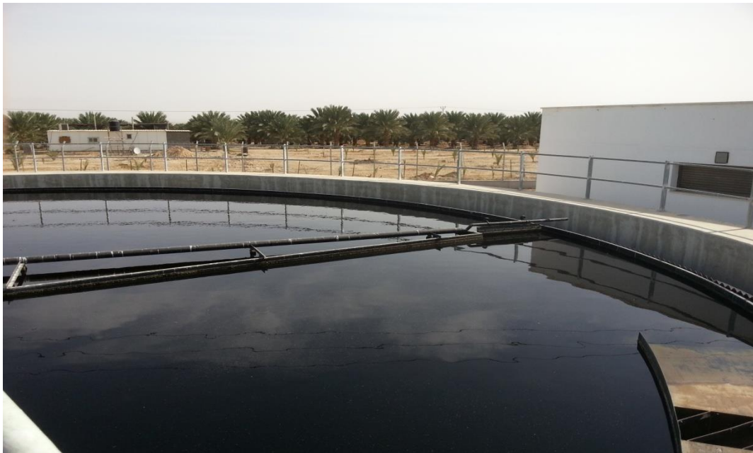
Figure (3.5): Clarifier in Jericho WWTP
