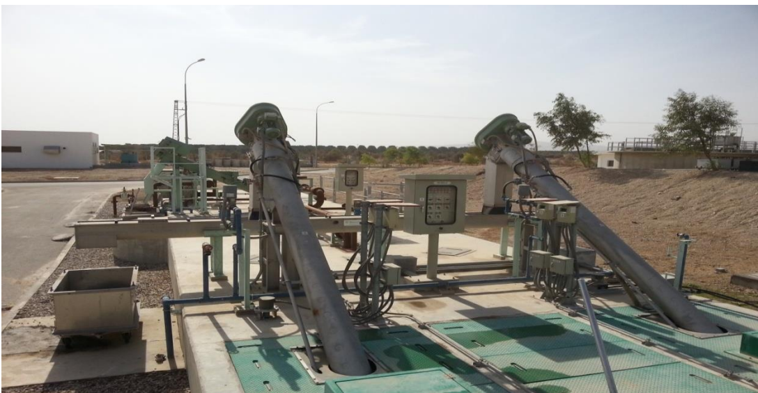
Figure (3.3): Screening in Jericho WWTP
